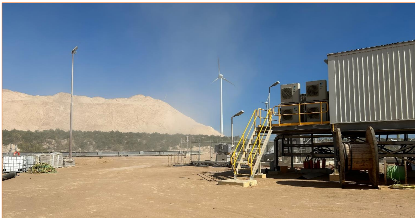
Figure 3-4: Air conditioners for the MCC are directly north of the tailings stockpile (ETA, 2023)
