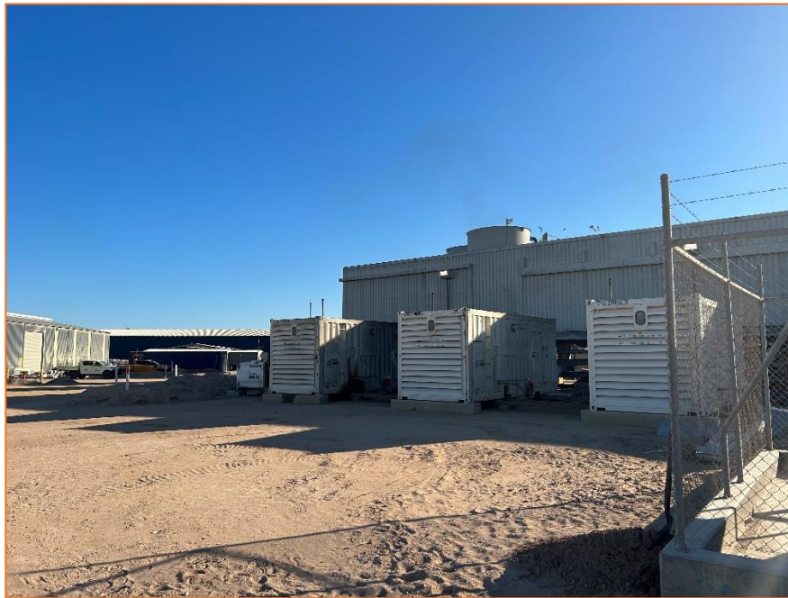
Figure 3-13: Diesel generators adjacent to MCC (ETA, 2023)
