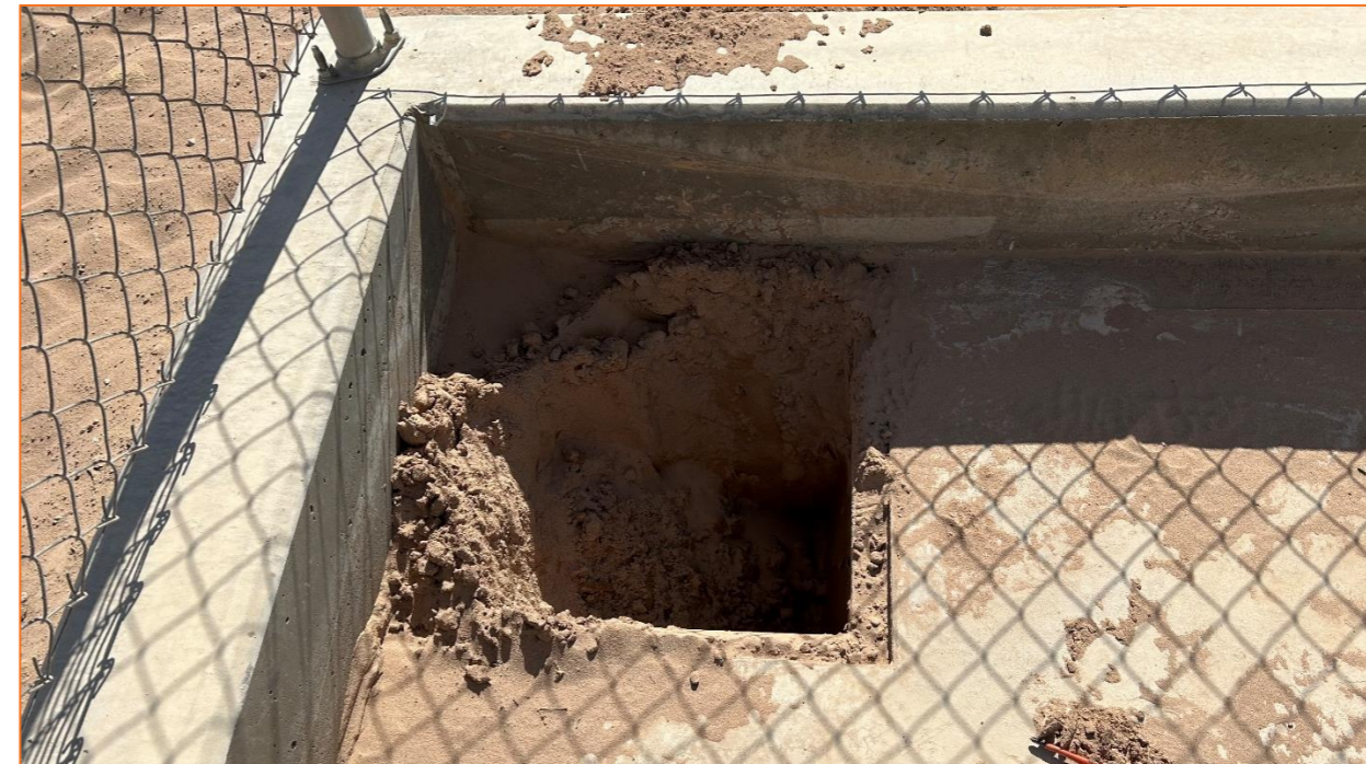
Figure 3-5: Recovery drain for potential oil spills from the transformers filled with sand (ETA, 2023)
