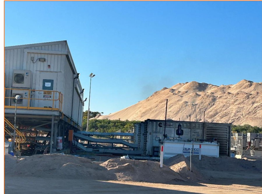
Figure 3-14: Diesel generators adjacent to MCC (ETA, 2023)
