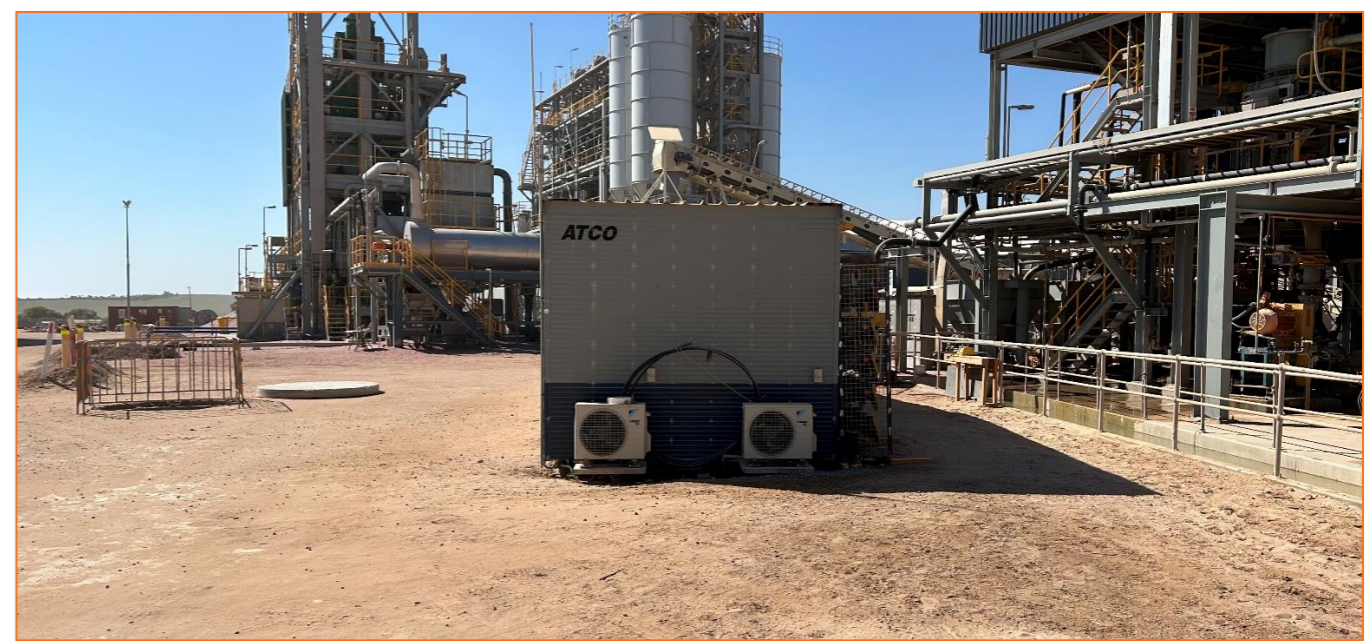
Figure 3-9 Air conditioners for control room at ground level (ETA, 2023)
