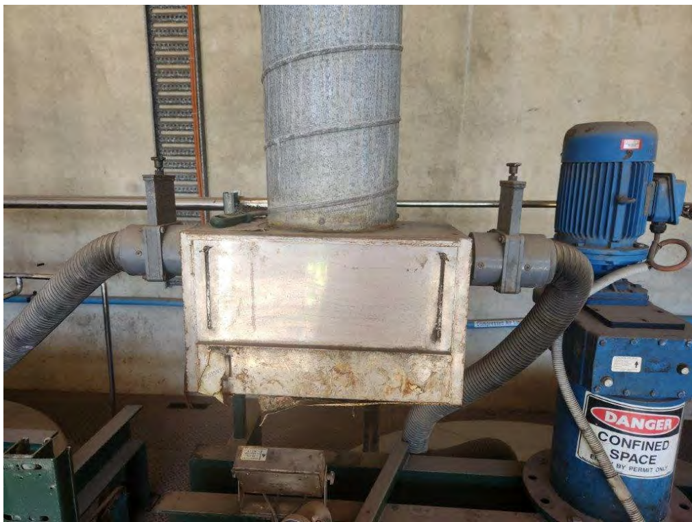
Figure 12: 61-F4 Plenum Chamber
