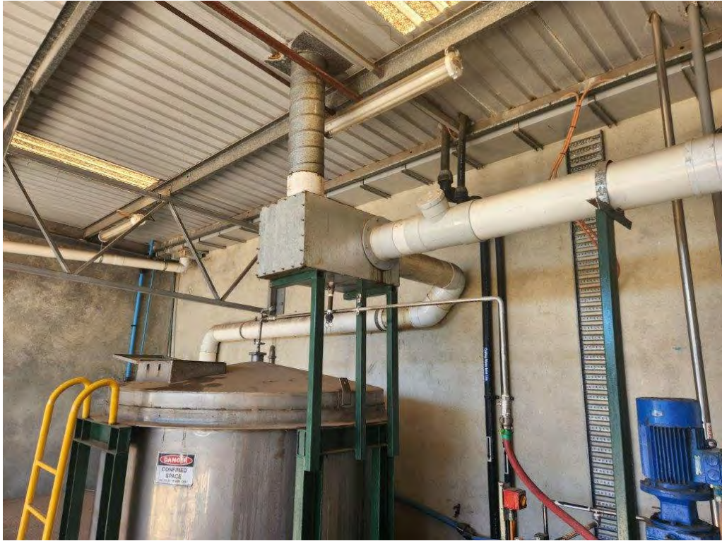
Figure 11: 61-F3 Plenum Chamber
