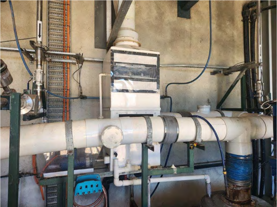
Figure 8: 61-F1 Wet Scrubber Gly
