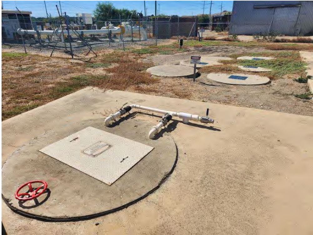
Figure 13: Stormwater Sullage pits
