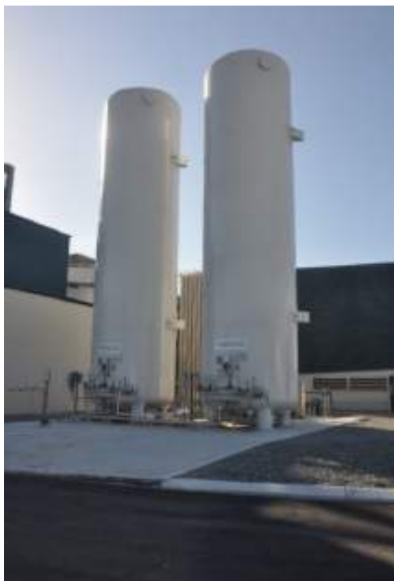
Plate 25 - Liquid Carbon Dioxide Storage Vessels (Southern Seawater Desalination Plant) (Northern Water Partnership, 2023)
