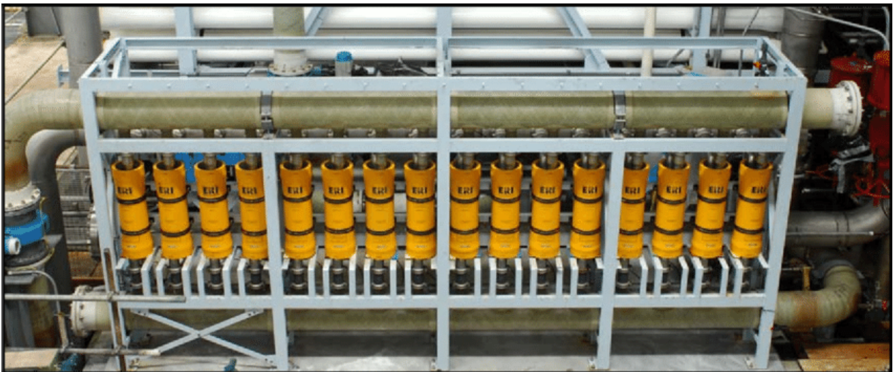
Plate 21 - Example of Typical RO Energy Recovery Rack within RO Building (Northern Water Partnership, 2023)
