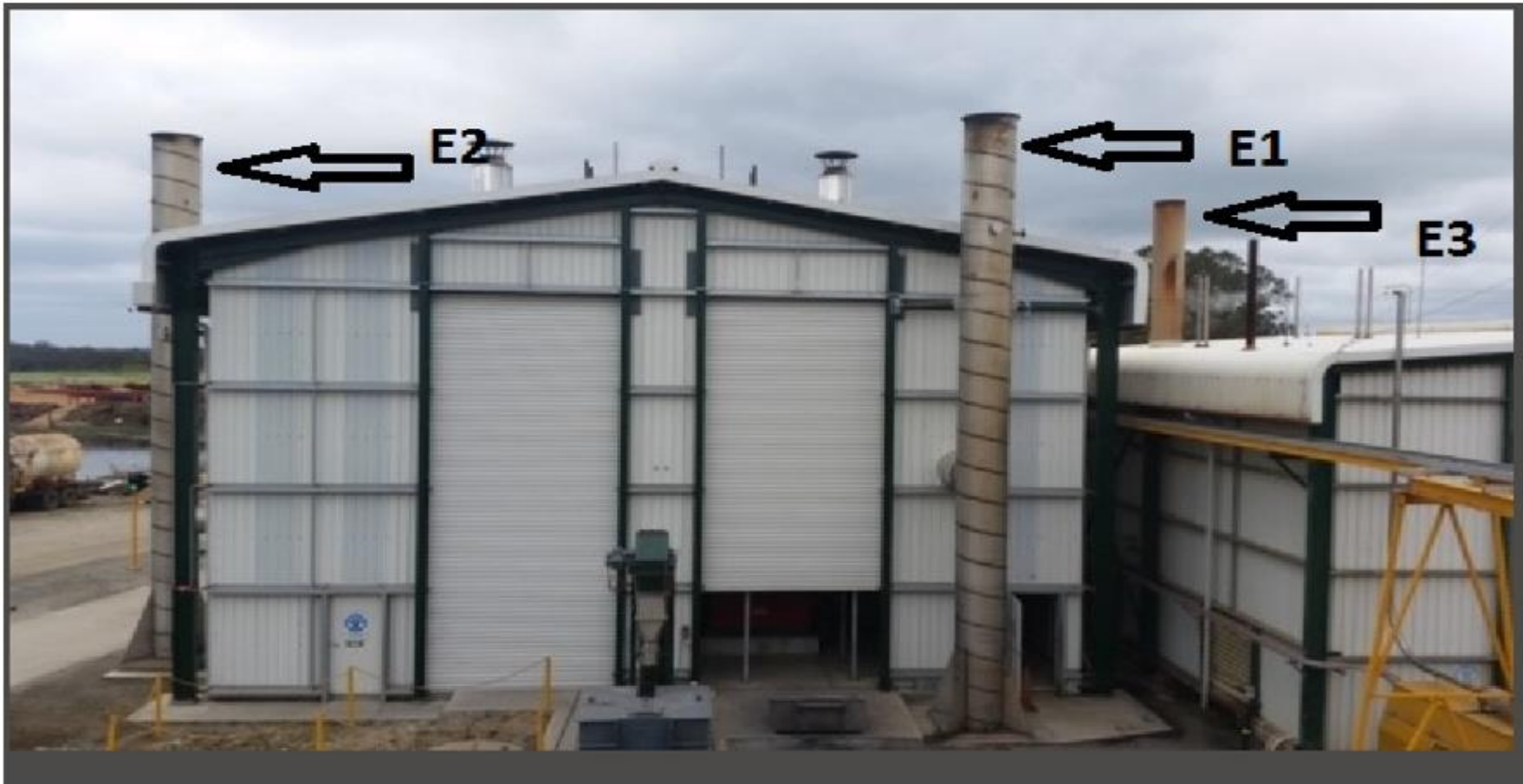
Figure 5: Biomass boilers emission points
