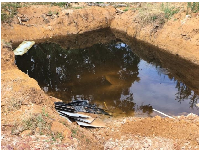
Photo 7 – Unburied asbestos material in asbestos disposal area.
