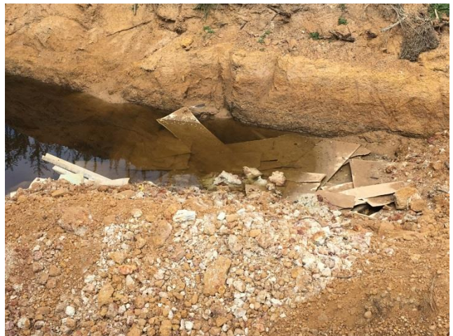
Photo 8 - Unburied asbestos material in asbestos disposal area.
