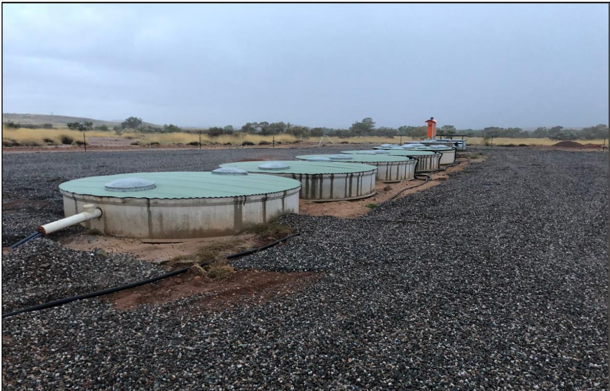
Figure 2: Biomax WWTP installed at the Premises
