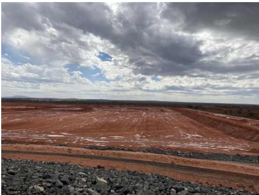
Plate 2: View of TSF-Cell 3 flooded working area.
