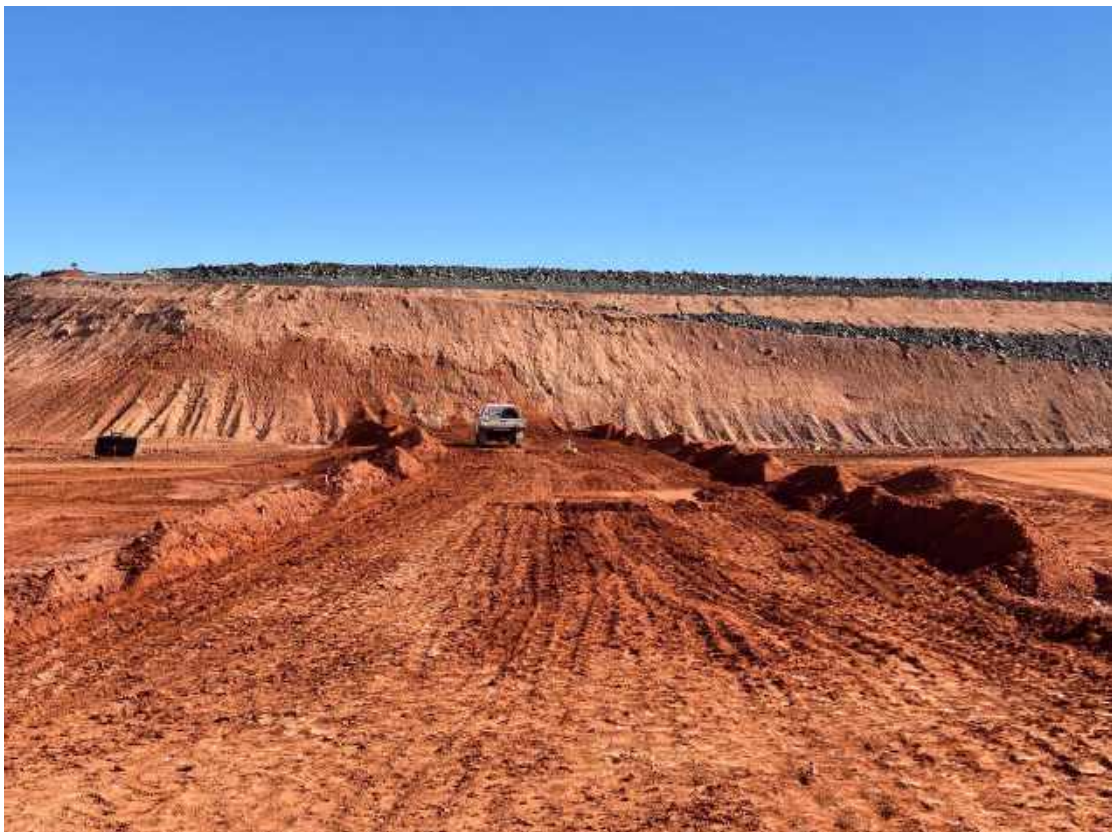
Plate 2: NDM Compaction test at South Embankment – Zone C – layer 3.
