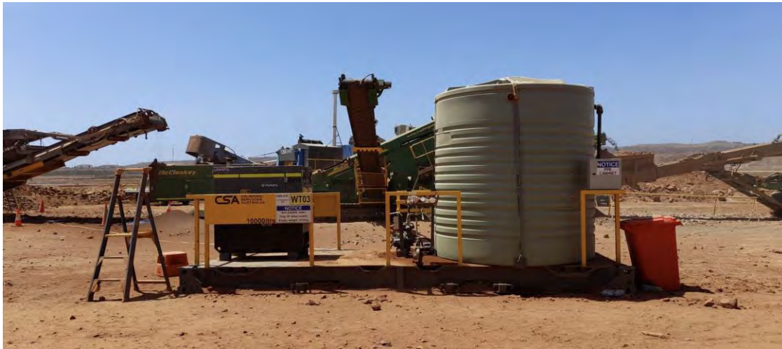
Figure 10 – Supporting infrastructure - 9,000 litre (L) dust suppression tank, with generator, that dust suppression equipment is supplied from.
