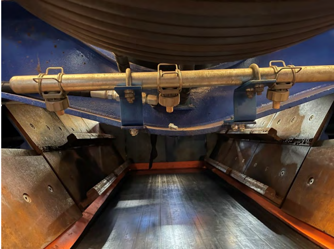
Figure 16 - Dust suppression sprays on Terex Pegson Maxtrak 1300 (secondary cone crusher) used on Sites C and F
