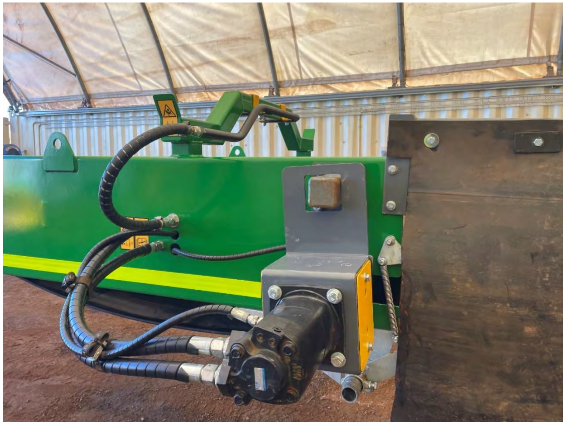
Figure 17 - KES 8048 Stacker Track Mounted (transfer conveyor) with dust suppression sprays on spray bar and transfer chute used on Sites C and F
