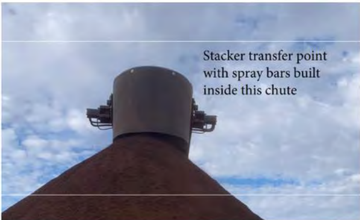
Figure 32 - Stacker transfer with dust controls
