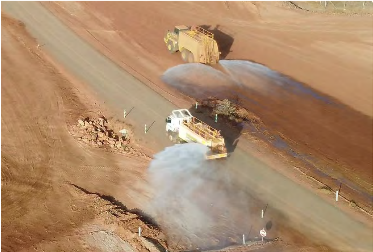
Figure 13 – The two different types of water carts in use, on Site C roads, 20 January 2024
