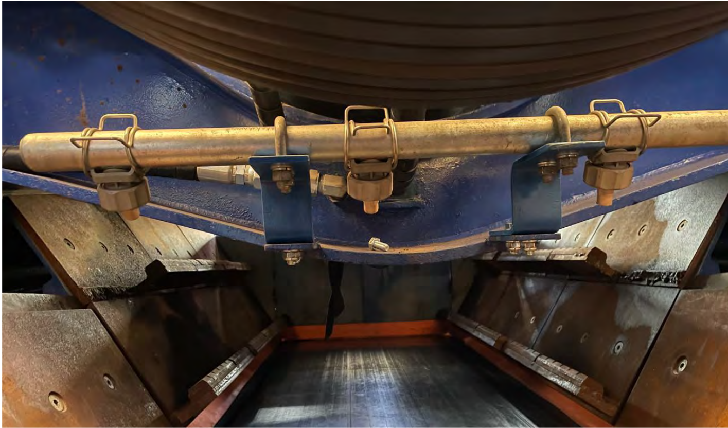
Figure 4-1 Dust Suppression Sprays Crusher Point
