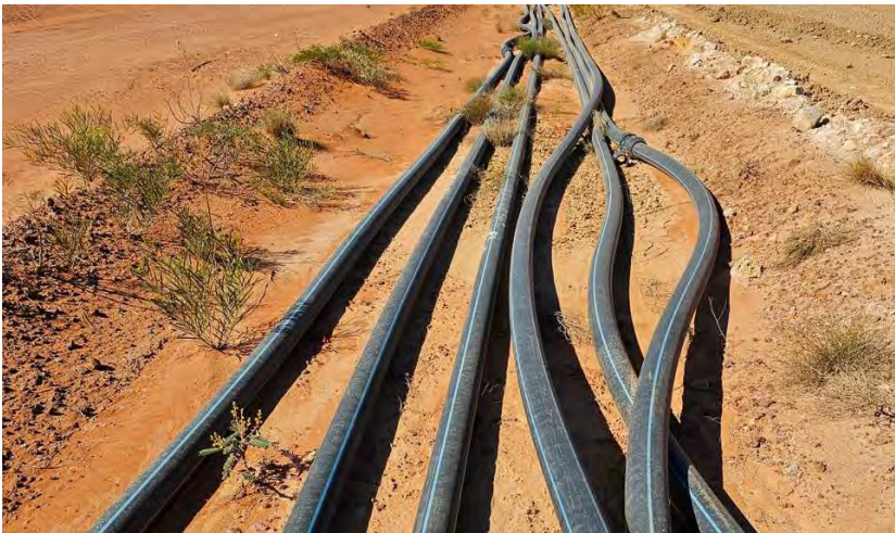
Figure 3: Photo showing pipelines (including dewatering) in v-drain (other pipelines carry water from supply bores)
