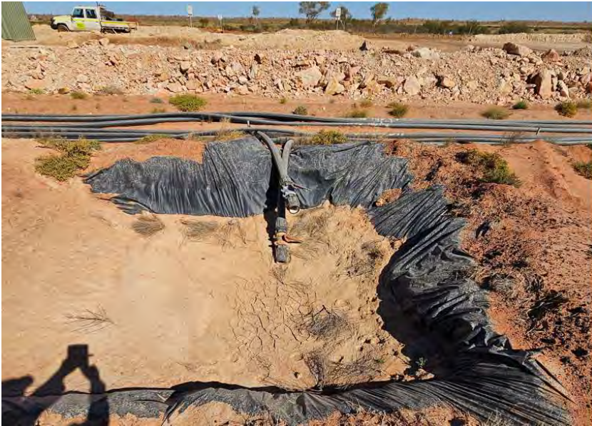
Figure 4: Photo showing pipelines (including dewatering), v-drain and lined overflow sump
