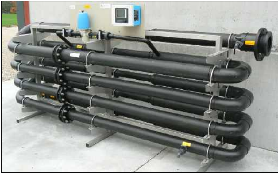
Plate 5-1: Typical neutralisation pipe reactor
