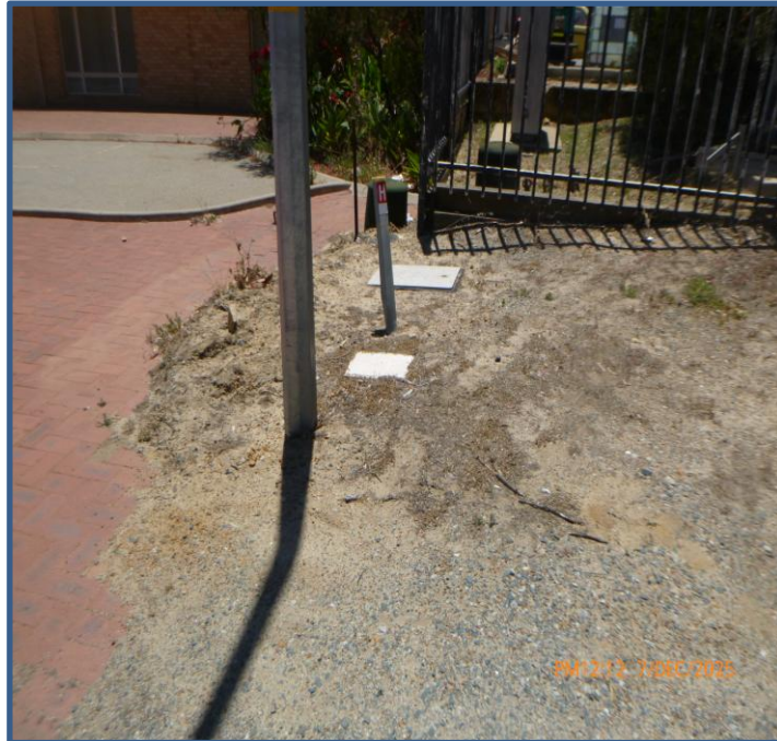
L 1: Street feed fire hydrant tested
