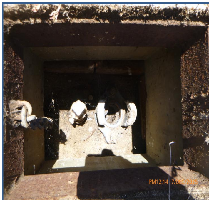
L 1: Internal view of street feed fire hydrant tested
