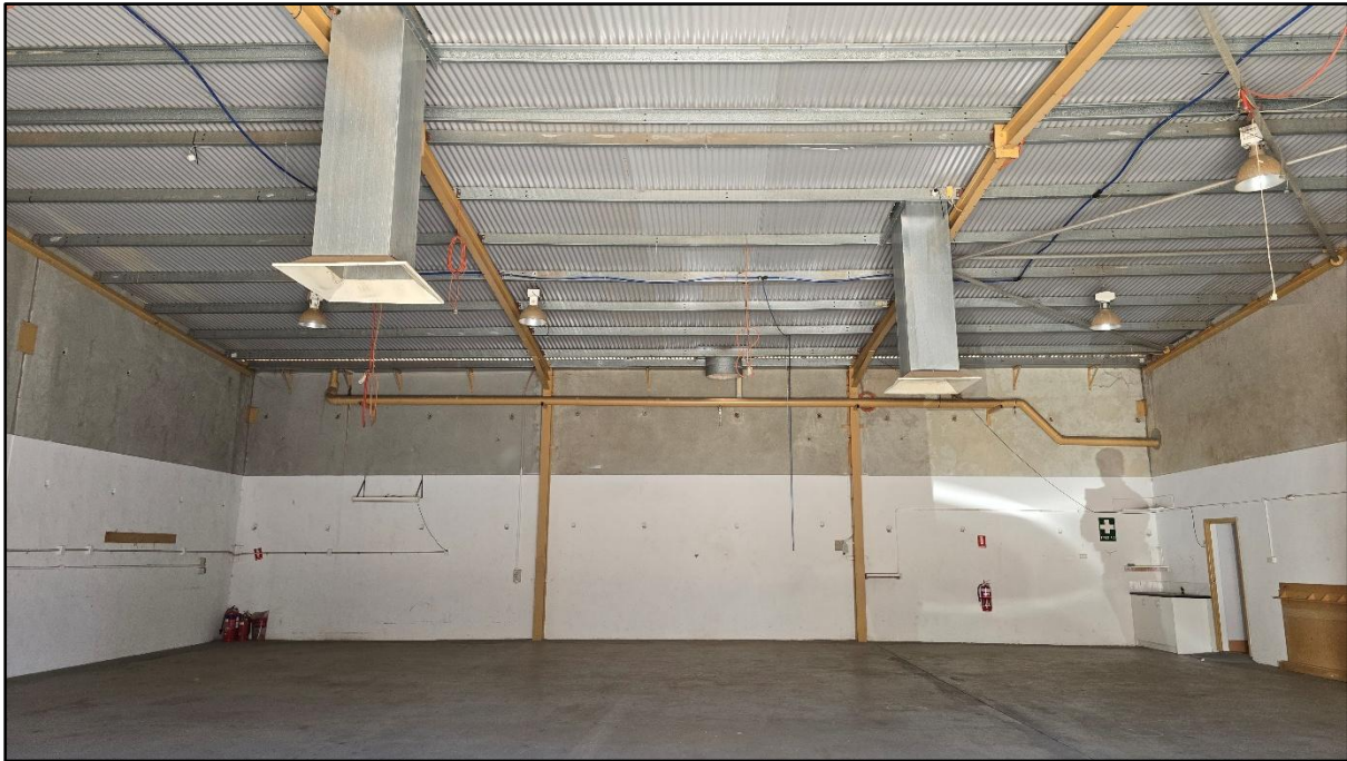
Figure 3-1: Photo of Existing Mechanical Ventilation Fans (West to East aspect)
