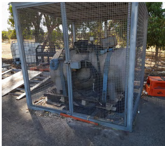
Existing fuel bowser and enclosure.
