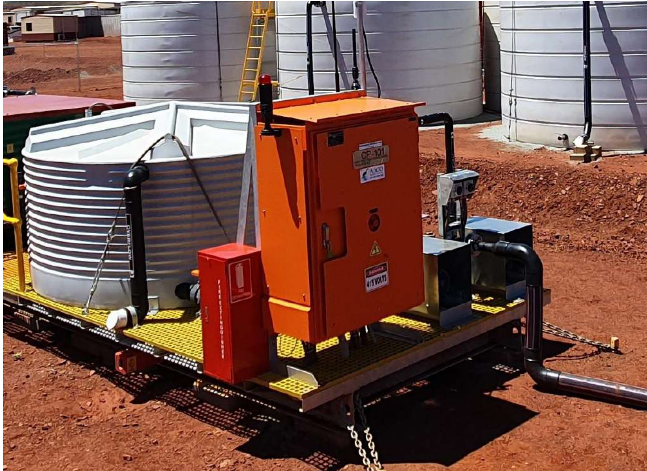
Figure 6: Evidence of Compliance – alarm system
