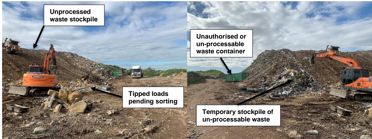
Figure 3: Tipped loads for sorting (left). Un-processable waste and container (right)
