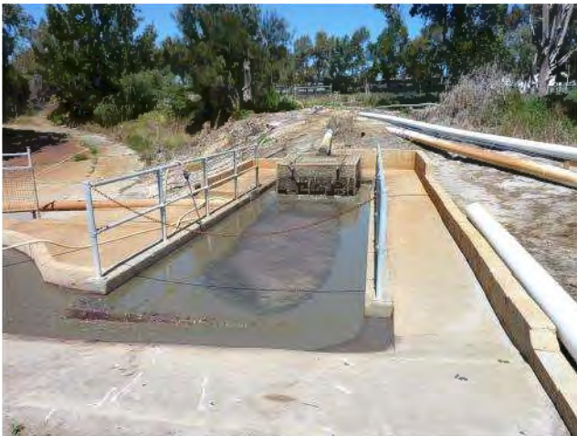
Photo 7 – WWTP inlet from conventional sheds showing gross solids cage
