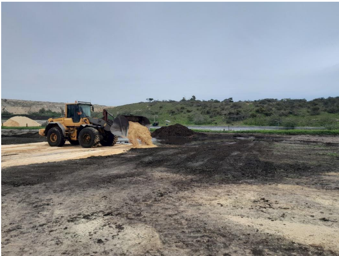
Figure 3 Limestone application in hardstand low points following removal of green waste mulch
