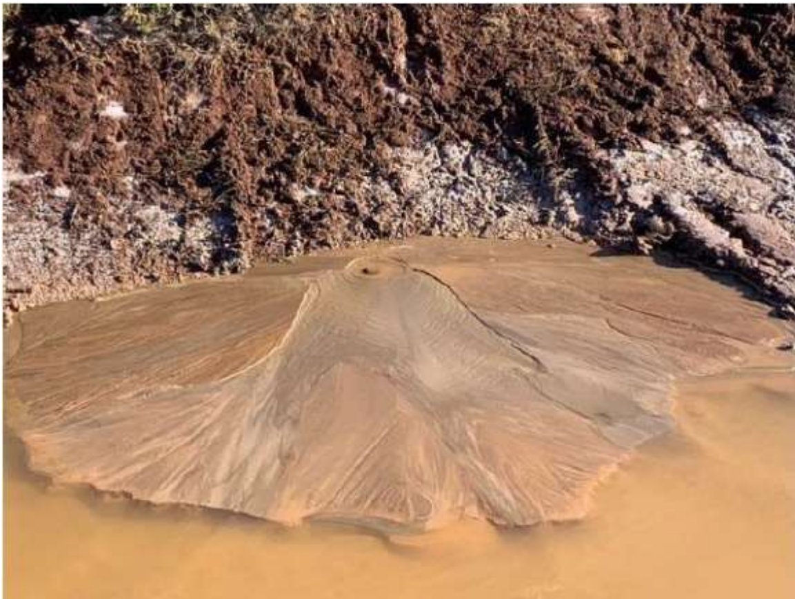
Figure 3: Sand boil in the toe drain near RB03 in January 2021 (Golders 2021, Sourced from Pennington Scott 2025)
