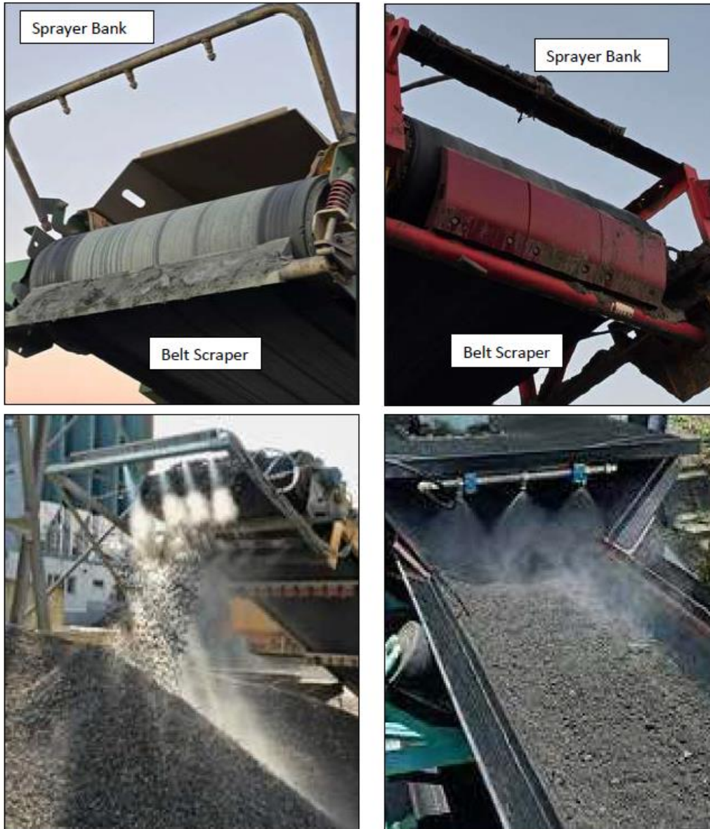
Figure 4: Crushing and Screening and DMS circuit sprayer examples
