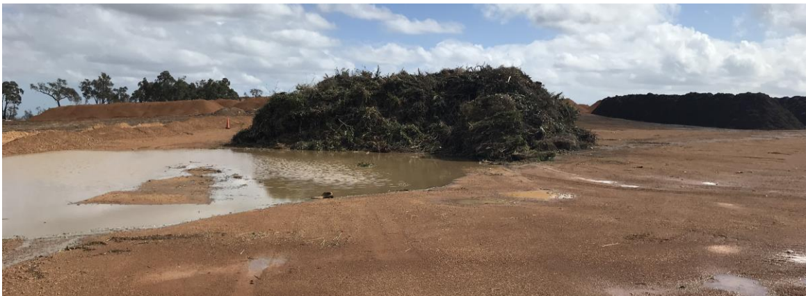
Figure 6: Stormwater/leachate pooling on the green waste processing hardstand, September 2019
