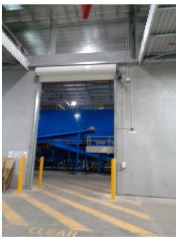
Photograph 4: Fire-rated walls and rapid close fire door separating the Production Area and Finished Product Store
