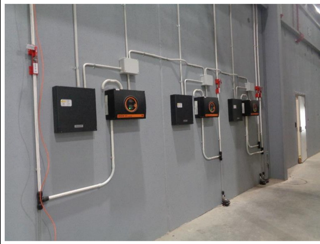
Photograph 3: Aspirating smoke detectors in the Finished Product Store
