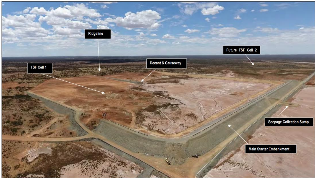
Figure 2: Seepage collection sump at the construction of TSF Cell 1 Stage 1 (Sourced from Dacian 2018)
