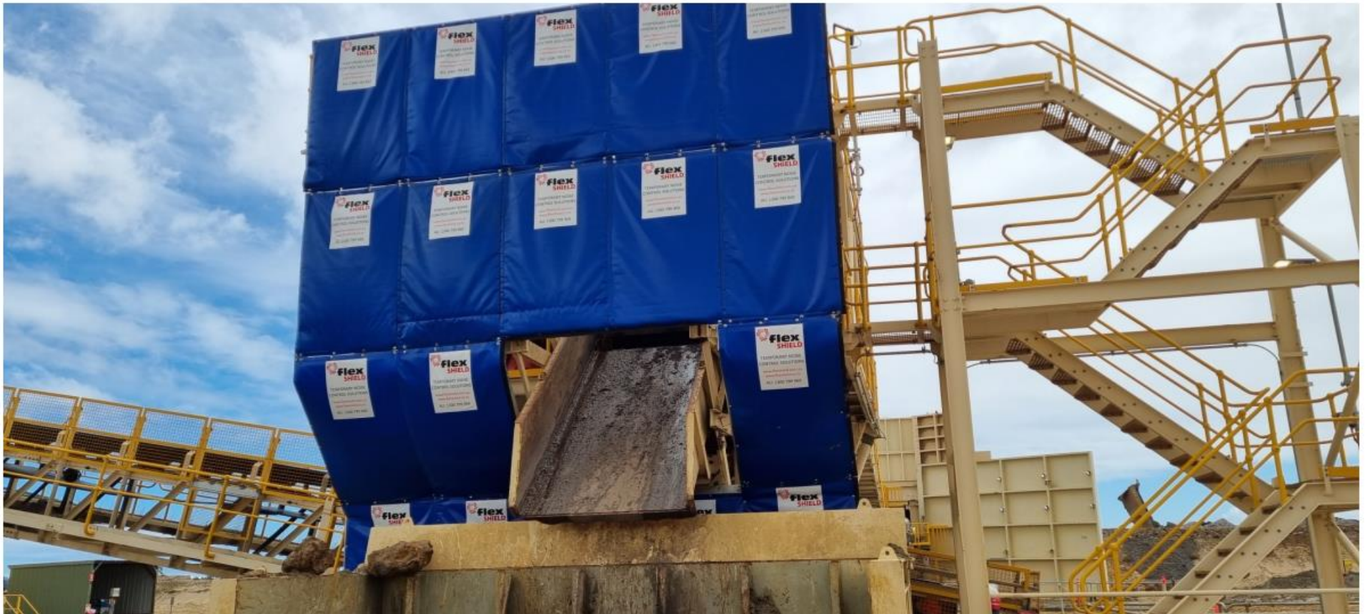
Plate 1: Sound suppression matting installed over the scalping screen.
