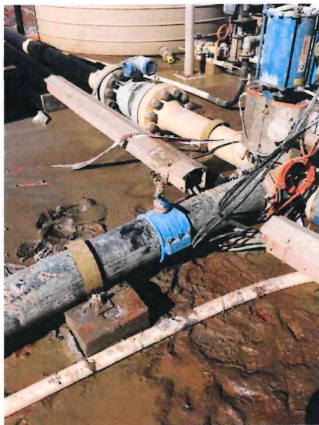
Figure 3- Saddle discharge location (saddle reinstated)
