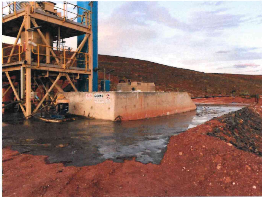
Figure 4- Paste Spill emergency bunker overwhelmed
