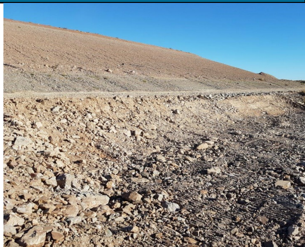
Plate 2 – Built up drain infrastructure (location of breach) front view of Plate 5 below.
