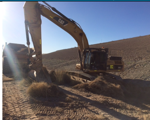
Plate 1 – Sediment basin constructed in front of toe drain (location of erosion breach).
