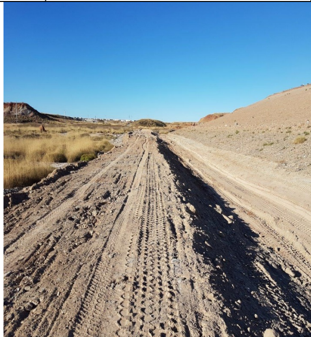
Plate 4 – Constructed bund and drain. Barrier to exclude further topsoil entering toe drain.
