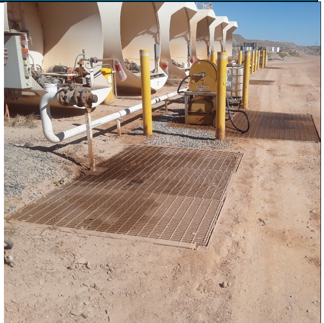
Plate 2 – Fuel farm after contaminated soil removed, signs of staining and potential contamination remain.
