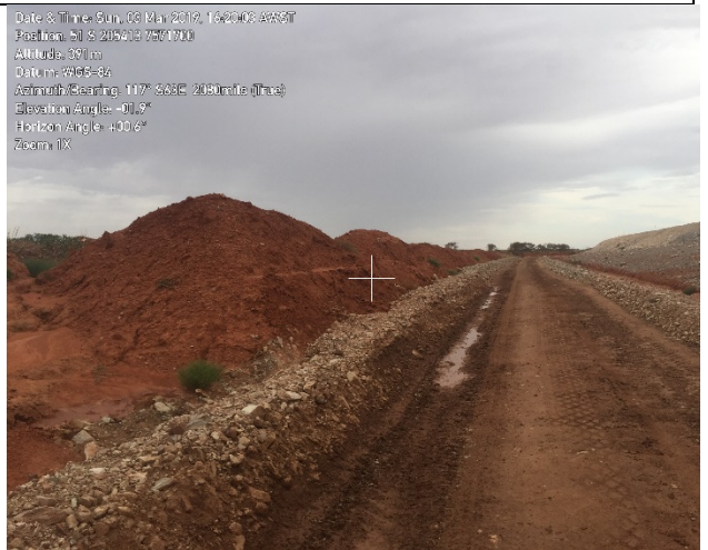
Plate 4 – Constructed bund and drain. Barrier to exclude further topsoil entering toe drain.
