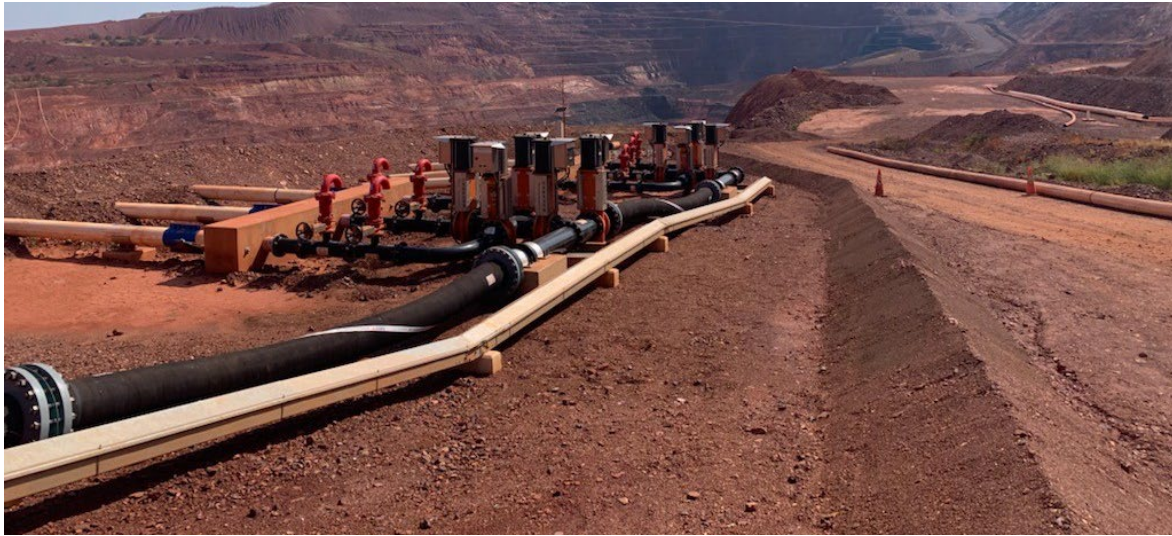
Figure I-1 Header Arrangement During Operation (No Leaks)
