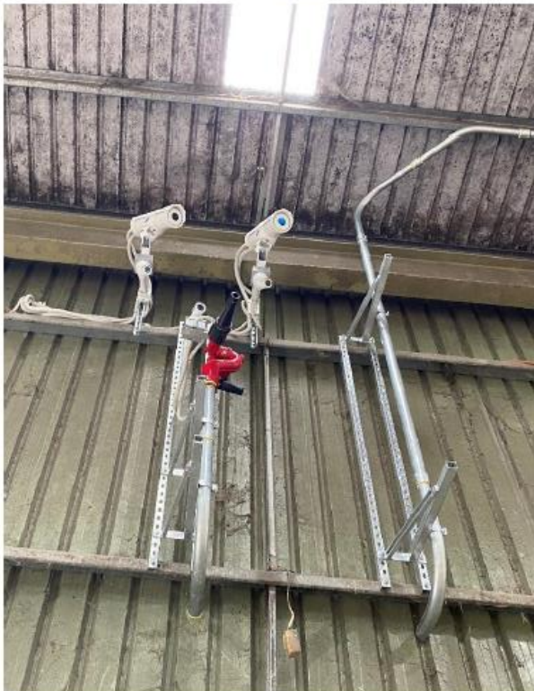
Figure 3.2 - FireRover Monitor and IR Cameras on Northern Wall looking from below
